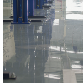
Epoxy and PU anti-static flooring
